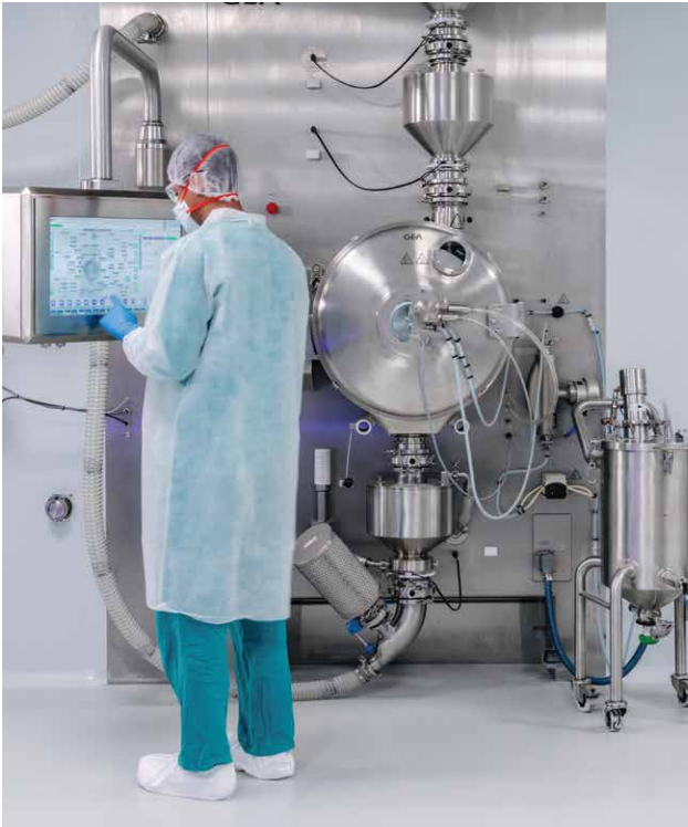
Hovione has installed state-of-the-art Continuous Tableting equipment
